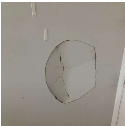
Comment: Hole in bedroom wall
