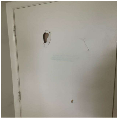
Comment: Hole in bedroom door
