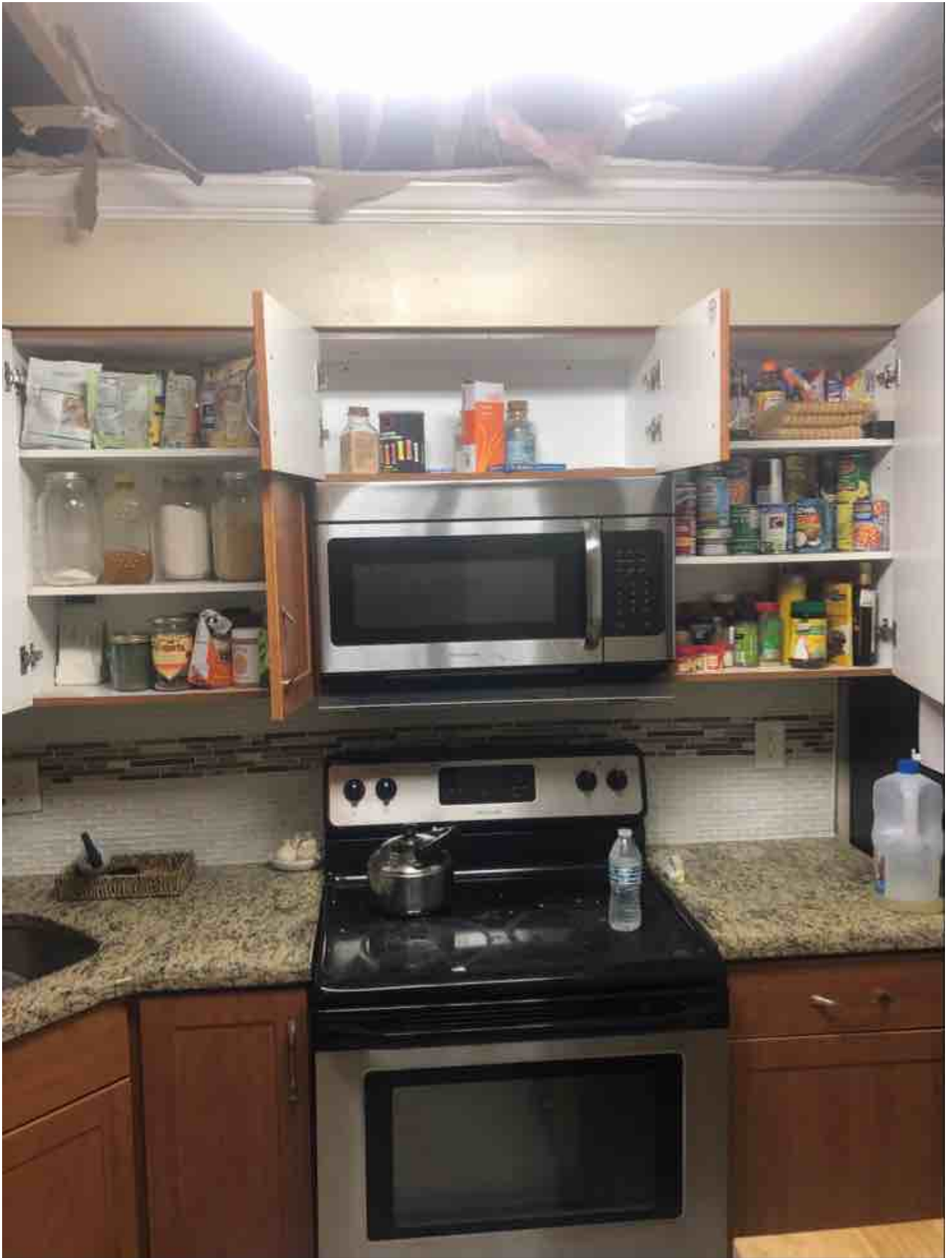
Cabinet Door: Not Ok
