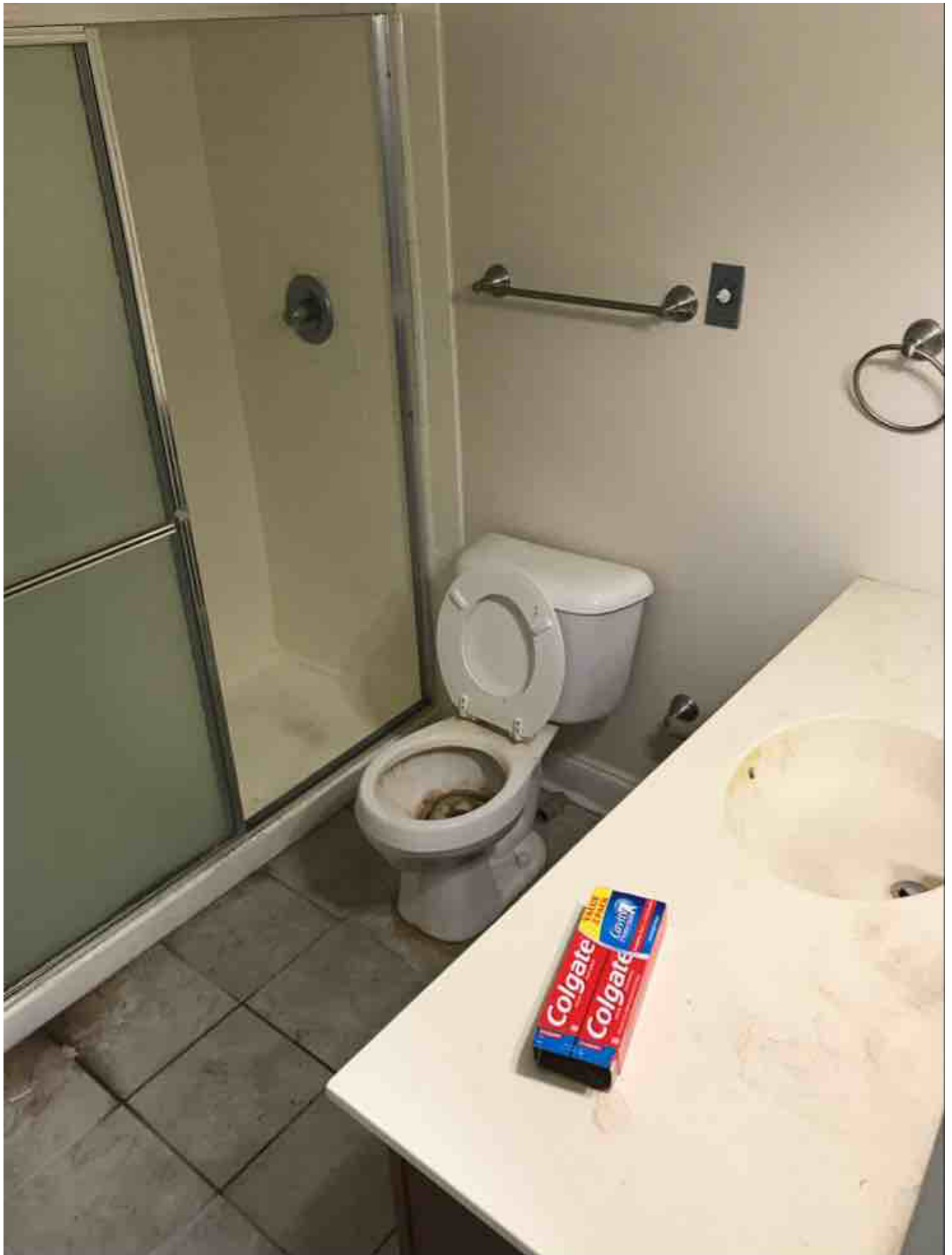
Cleaning Bathroom: Not Ok
