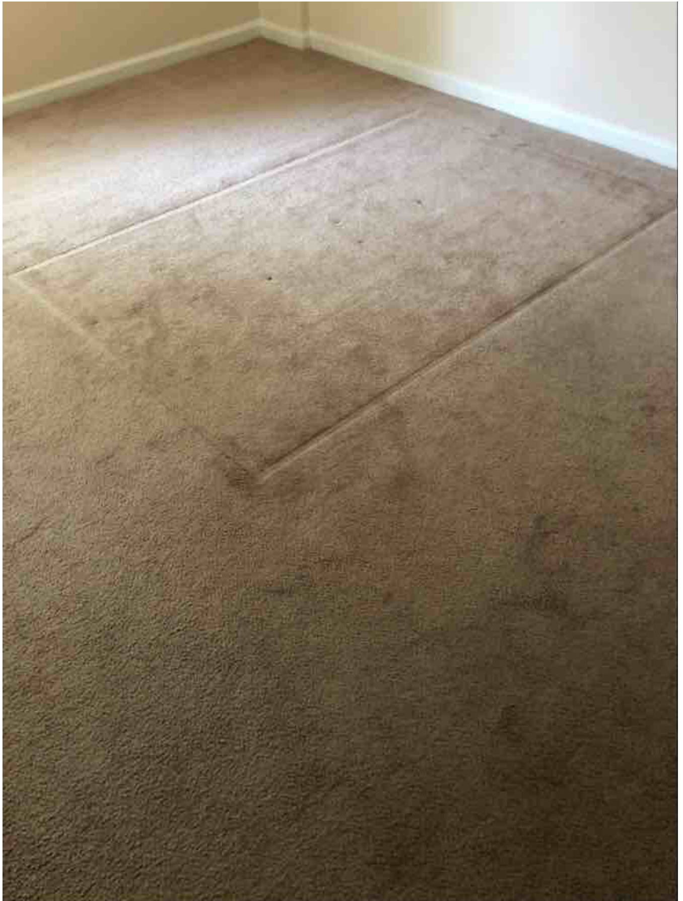
Stain Removal: Not Ok
