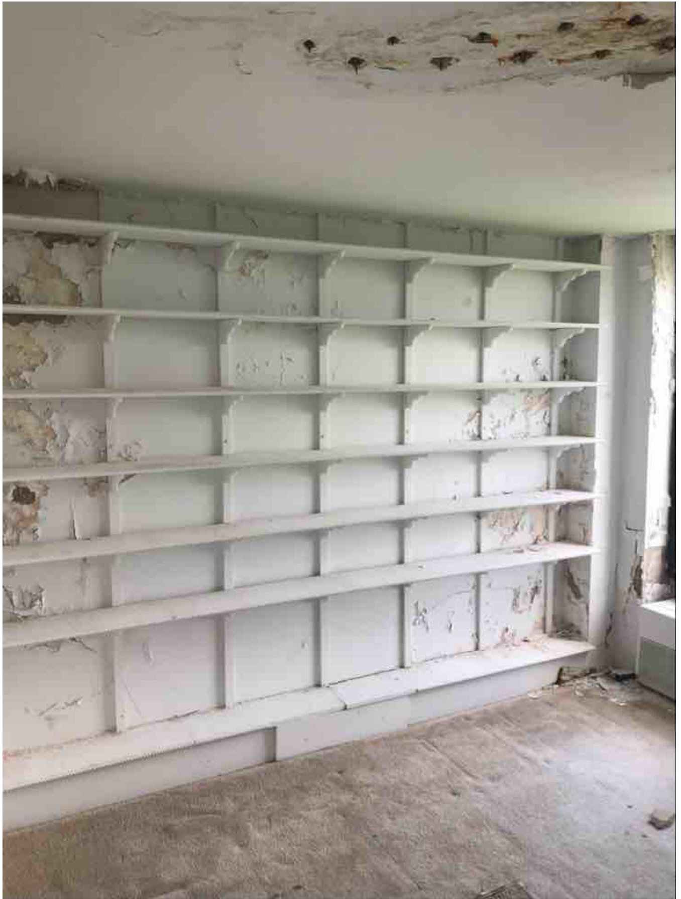
Ceilings / Lights: Not Ok
