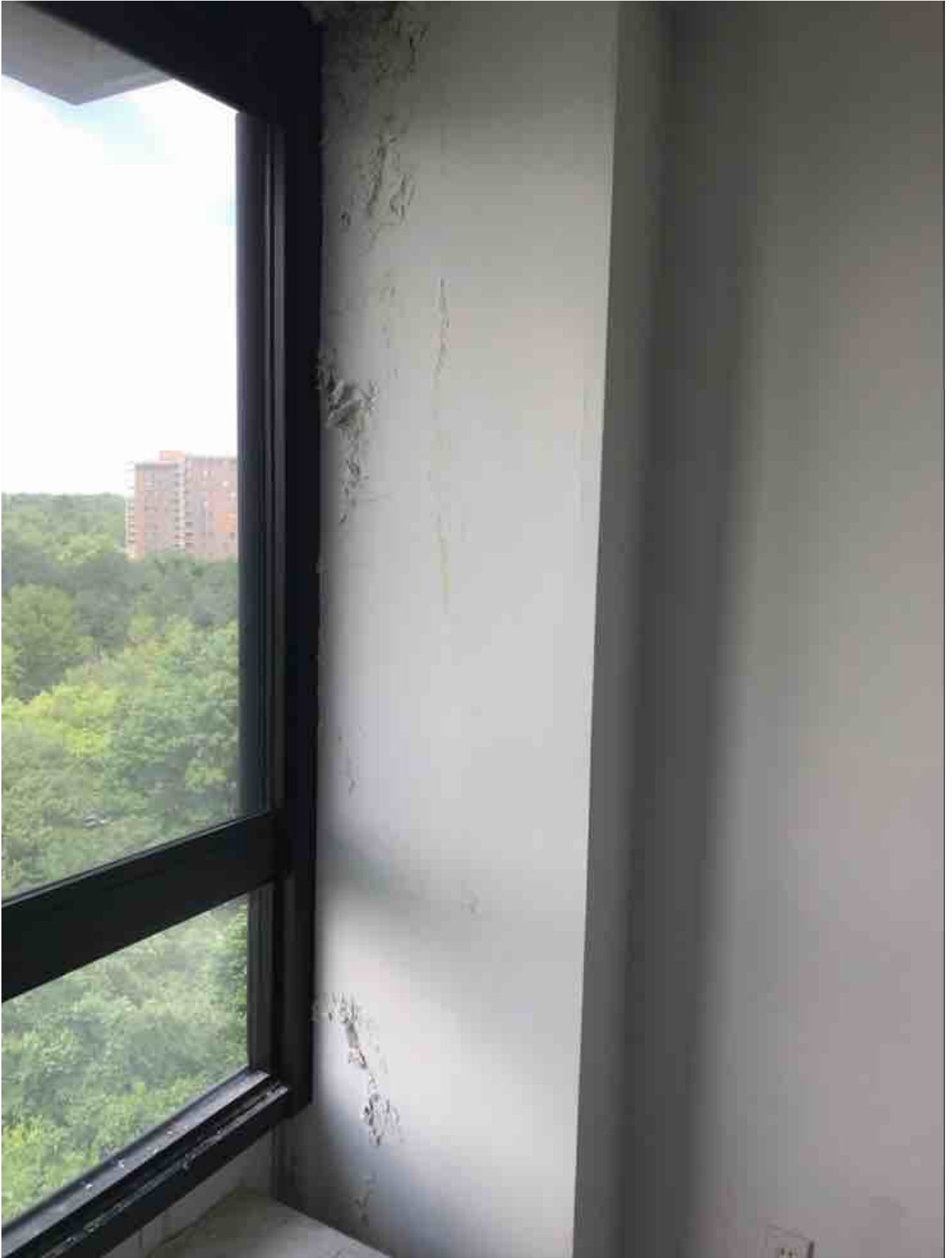
Ceilings / Lights: Not Ok
