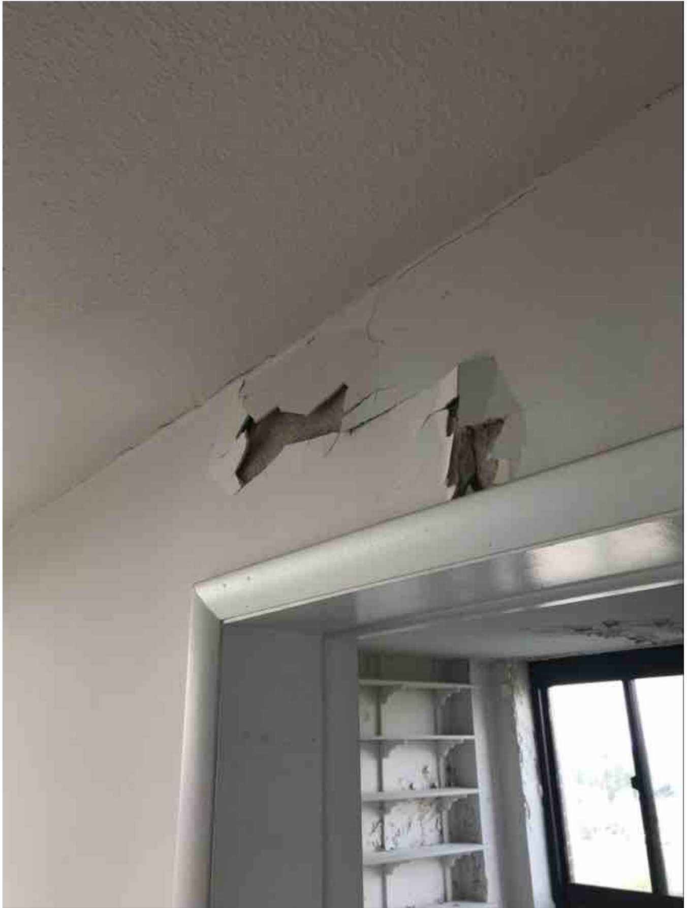
Walls / Outlets: Not Ok
