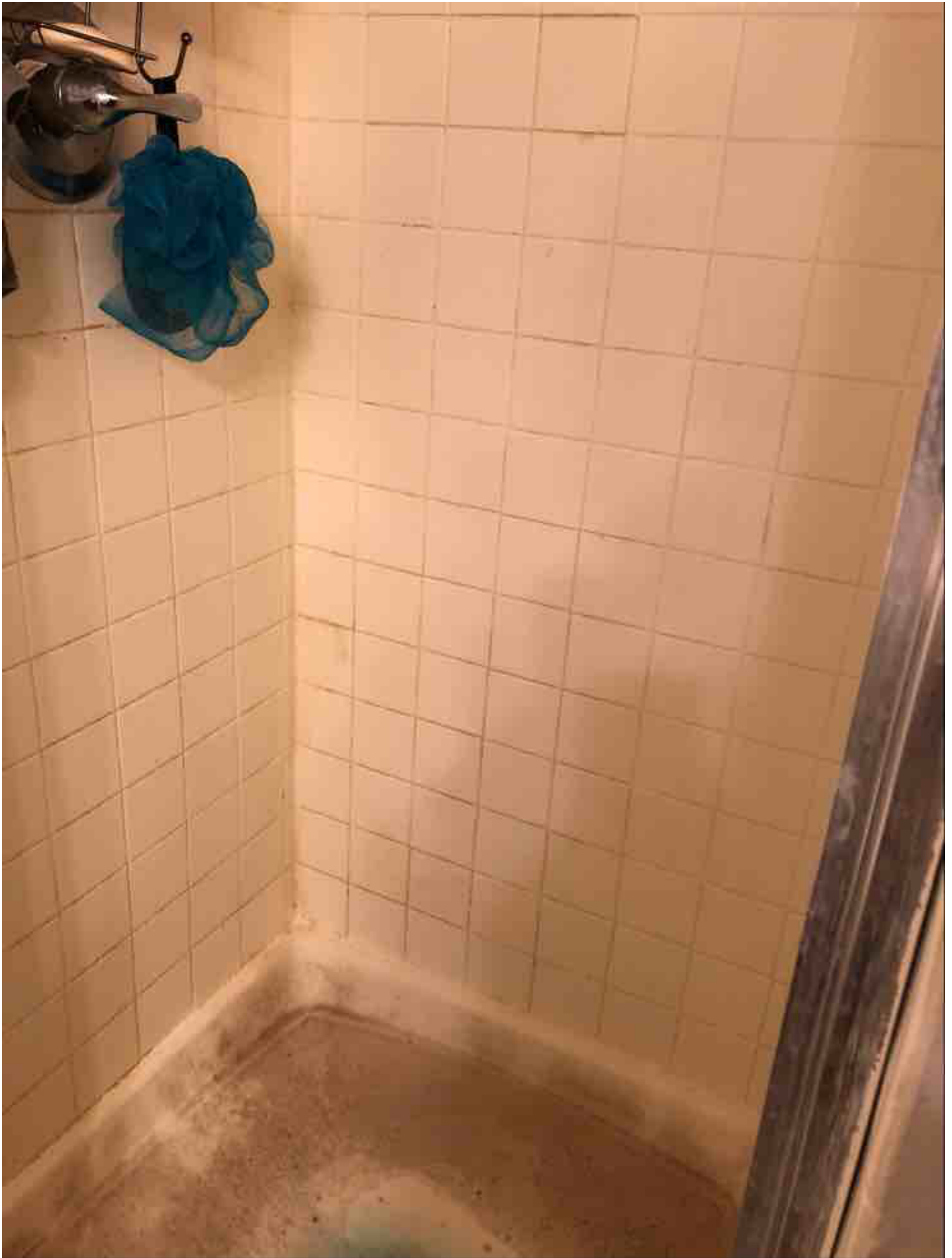
Cleaning Bathroom: Not Ok
