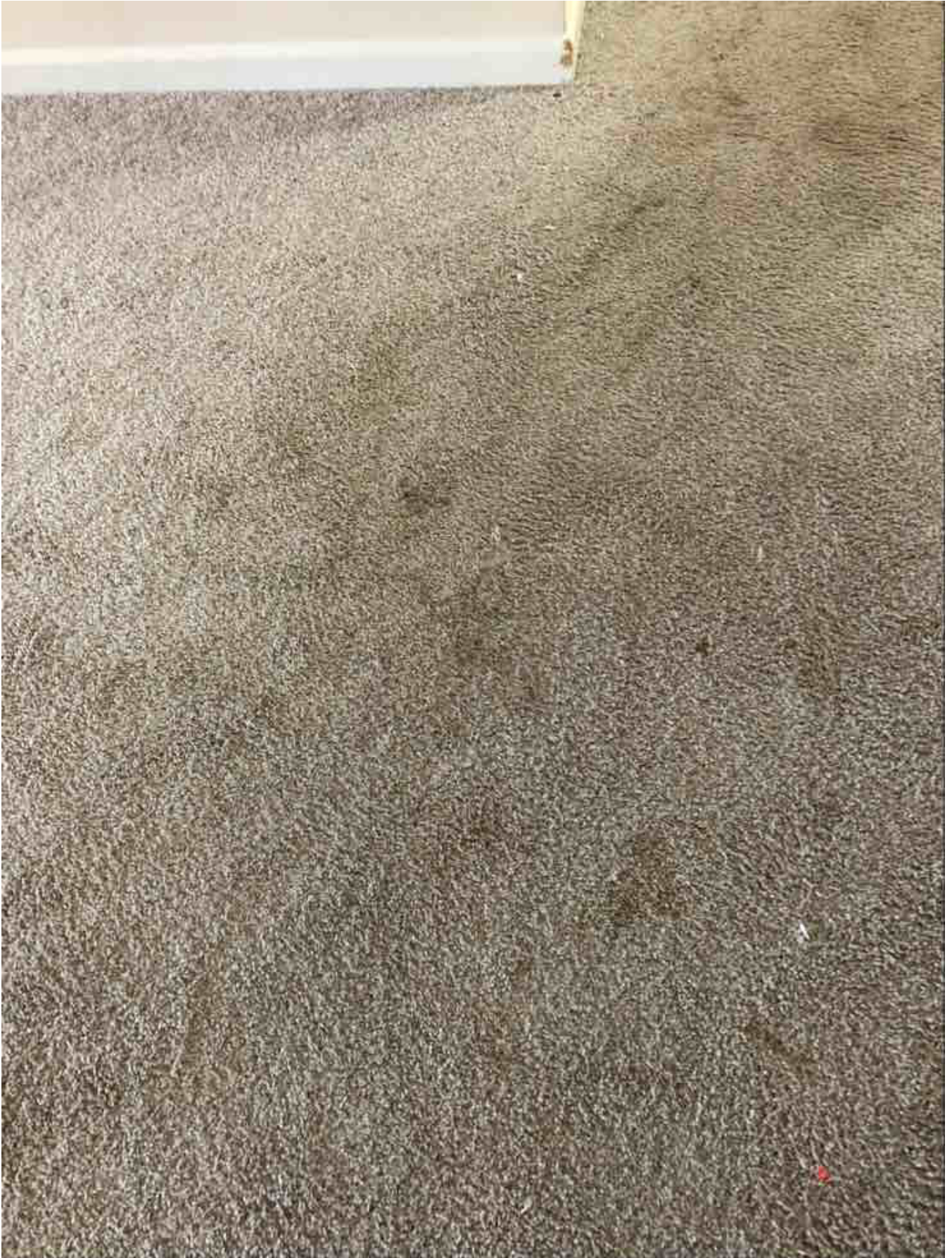
Stain Removal: Not Ok
