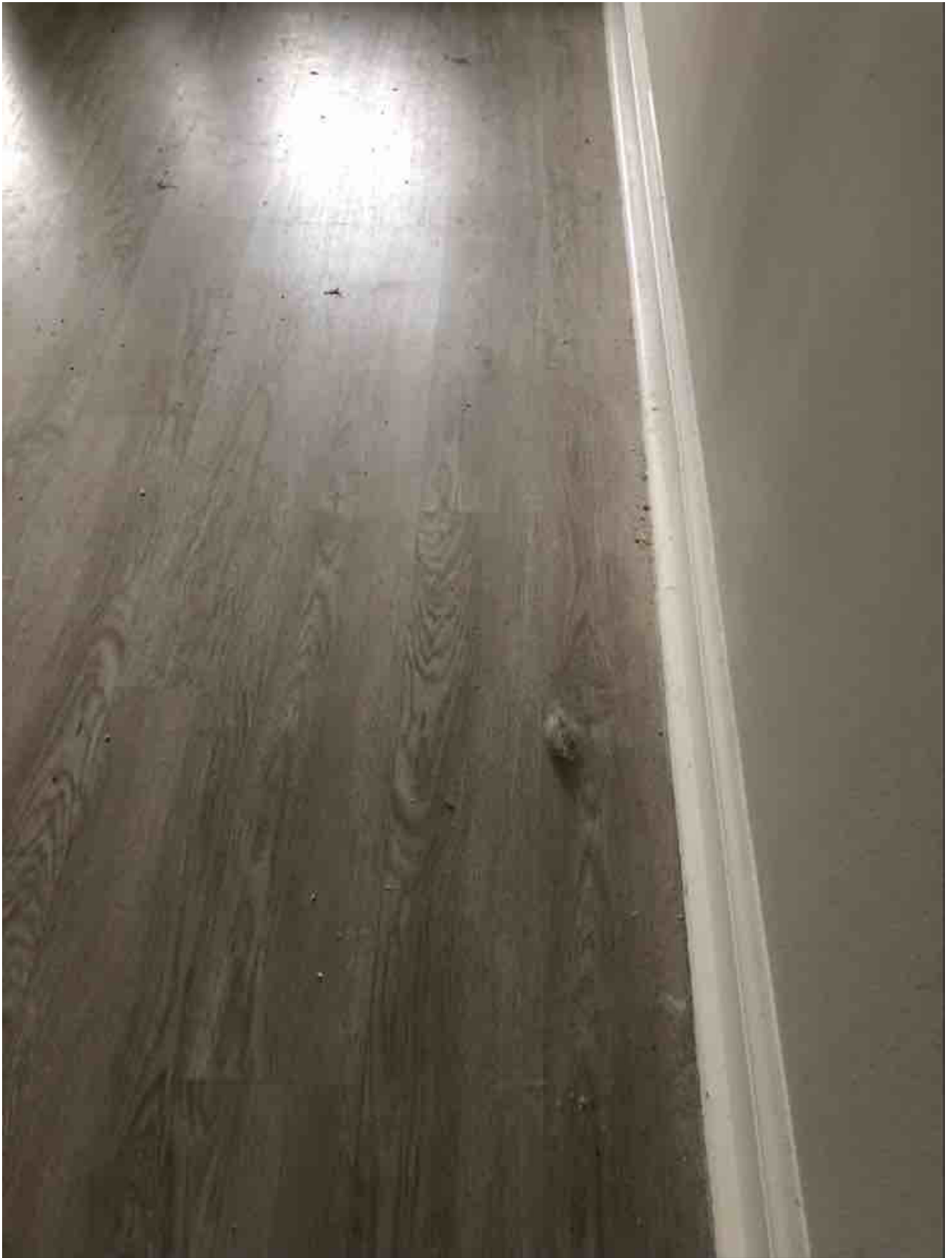
Closets cleared: Not Ok
