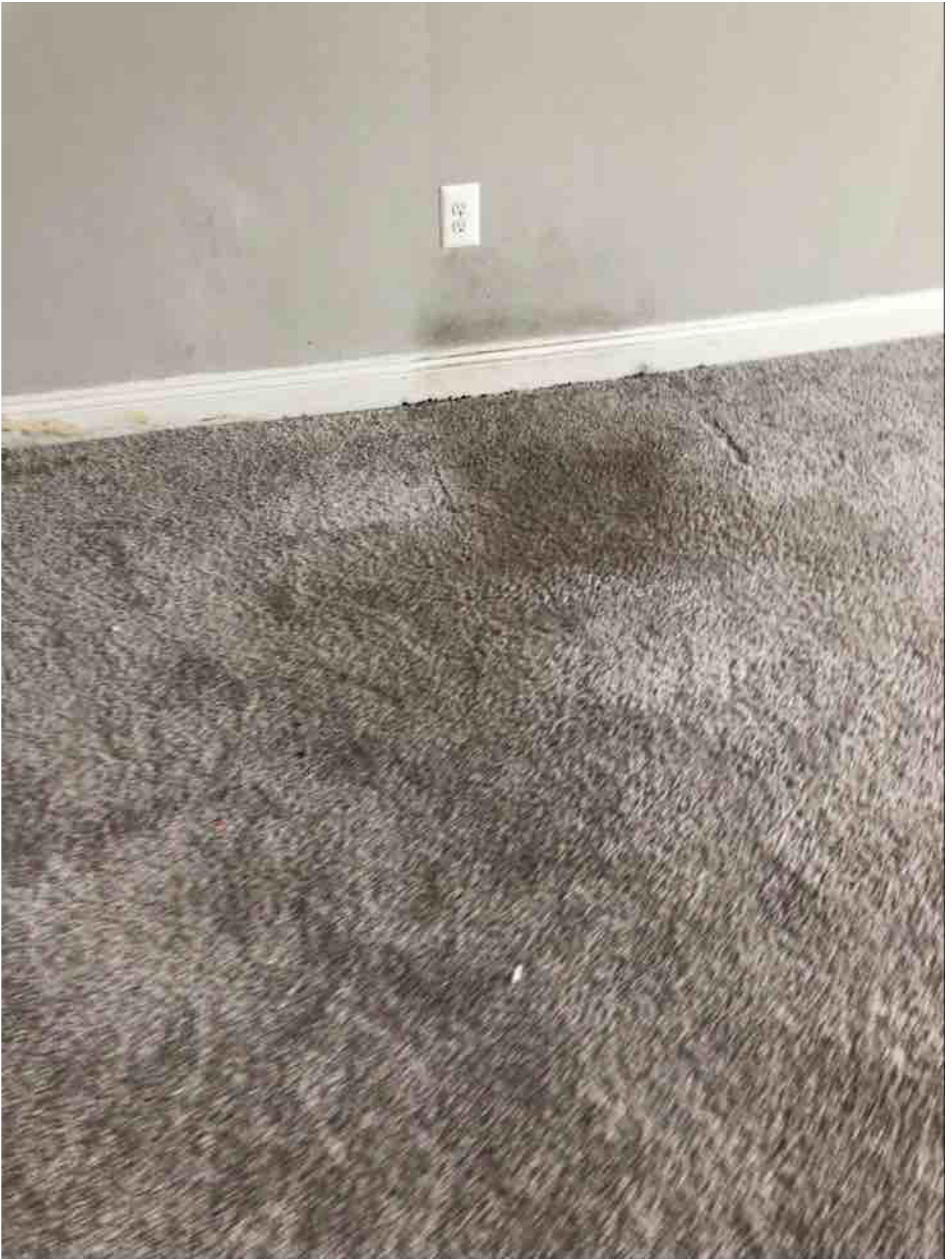
Stain Removal: Not Ok
