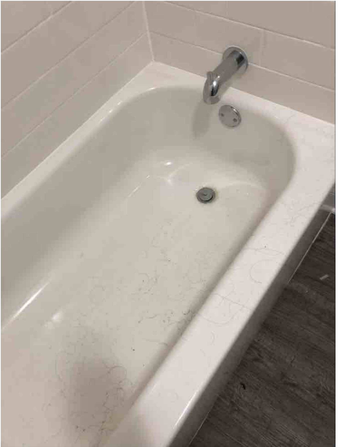
Cleaning Bathroom: Not Ok
